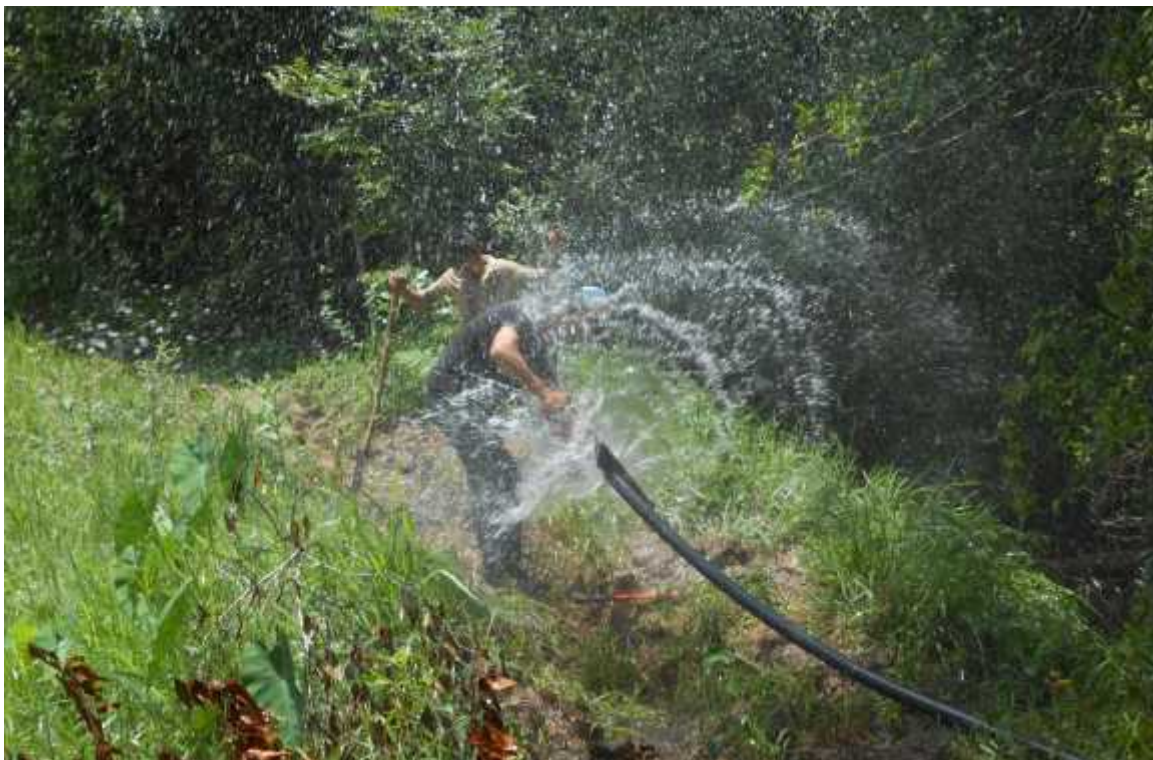
Me attending to a small leak.
