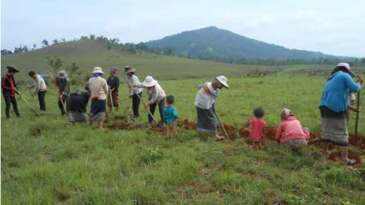
Mostly ladies starting to dig a 4 km long pipe trench. Note that the lady in the middle of the picture has her baby on her back. The men were away planting rice.
